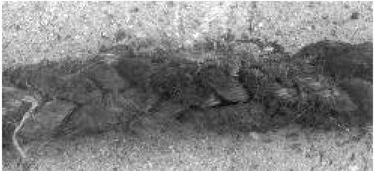
Figure D-006 Extensive External Abrasion
